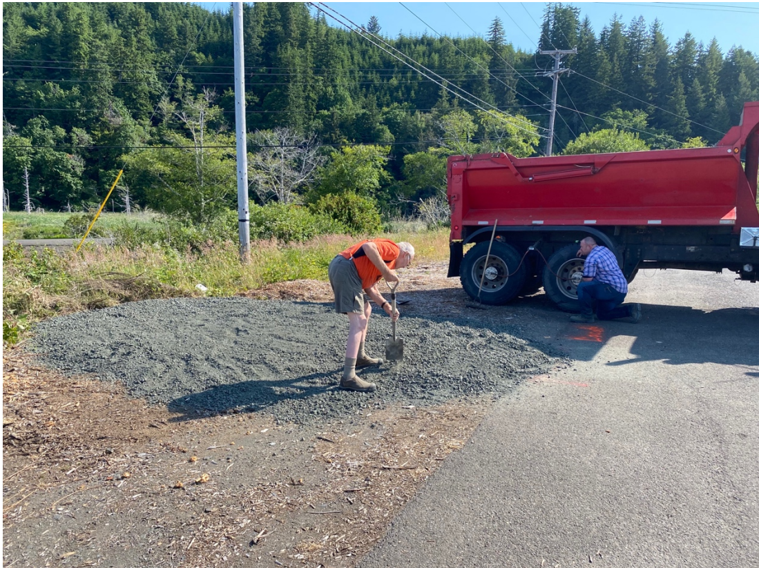
Chris Williams, truck driver for Coos Bay Timber Operators, takes a break while observing David Gould putting finishing touches on leveling gravel base for the Memorial stone near Stables Road entrance to Lower Smith River Road, Douglas County, Oregon, June 21, 2023.
