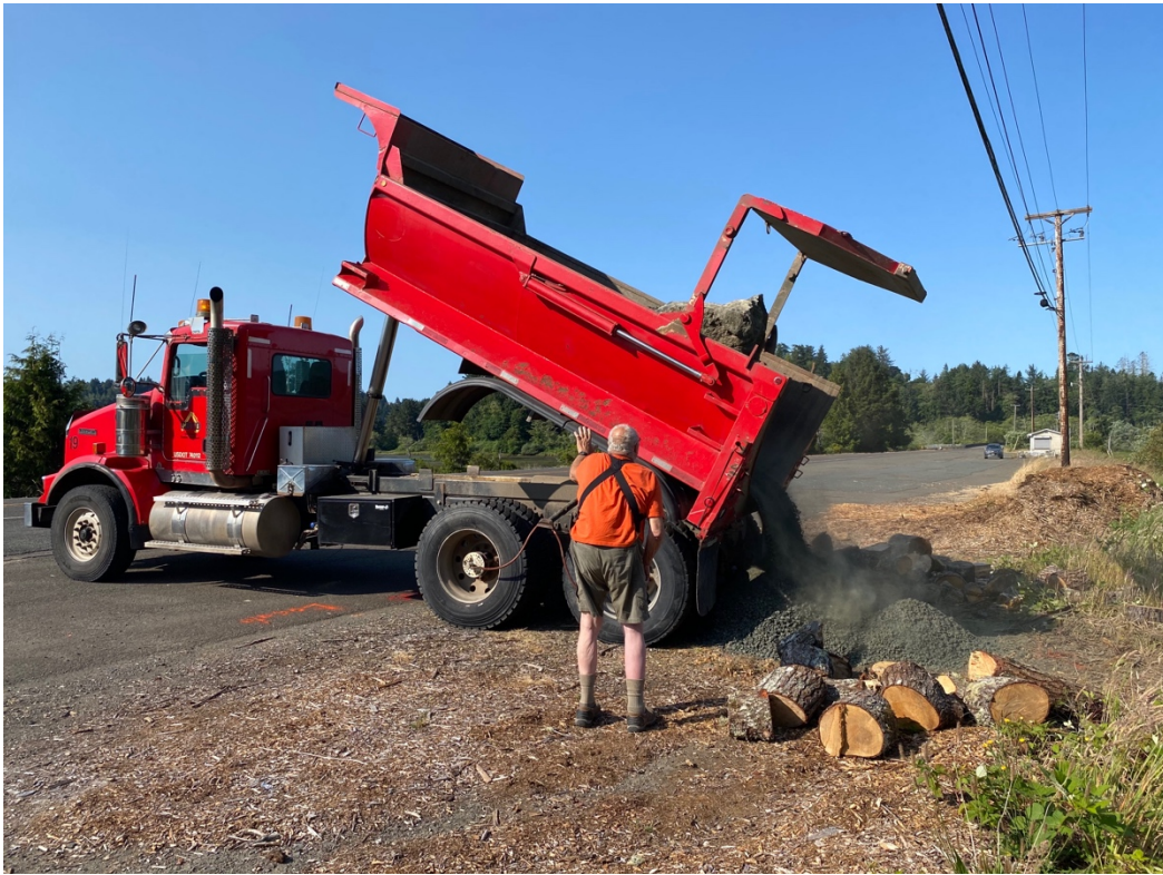
David Gould directs Coos Bay Timber Operators truck driver, Chris Williams, into dumping of gravel and Memorial stone at destination of Smith River mouth on the Umpqua River, in Douglas County, Oregon, June 21, 2023.
