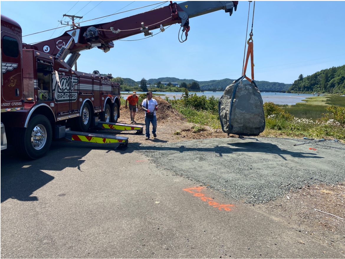
David Gould, Coos Bay Timber Operators, watches as Josh Mast, Mast Brothers, moves Memorial stone into its permanent location near the mouth of Smith River, Oregon, June 21, 2023.
