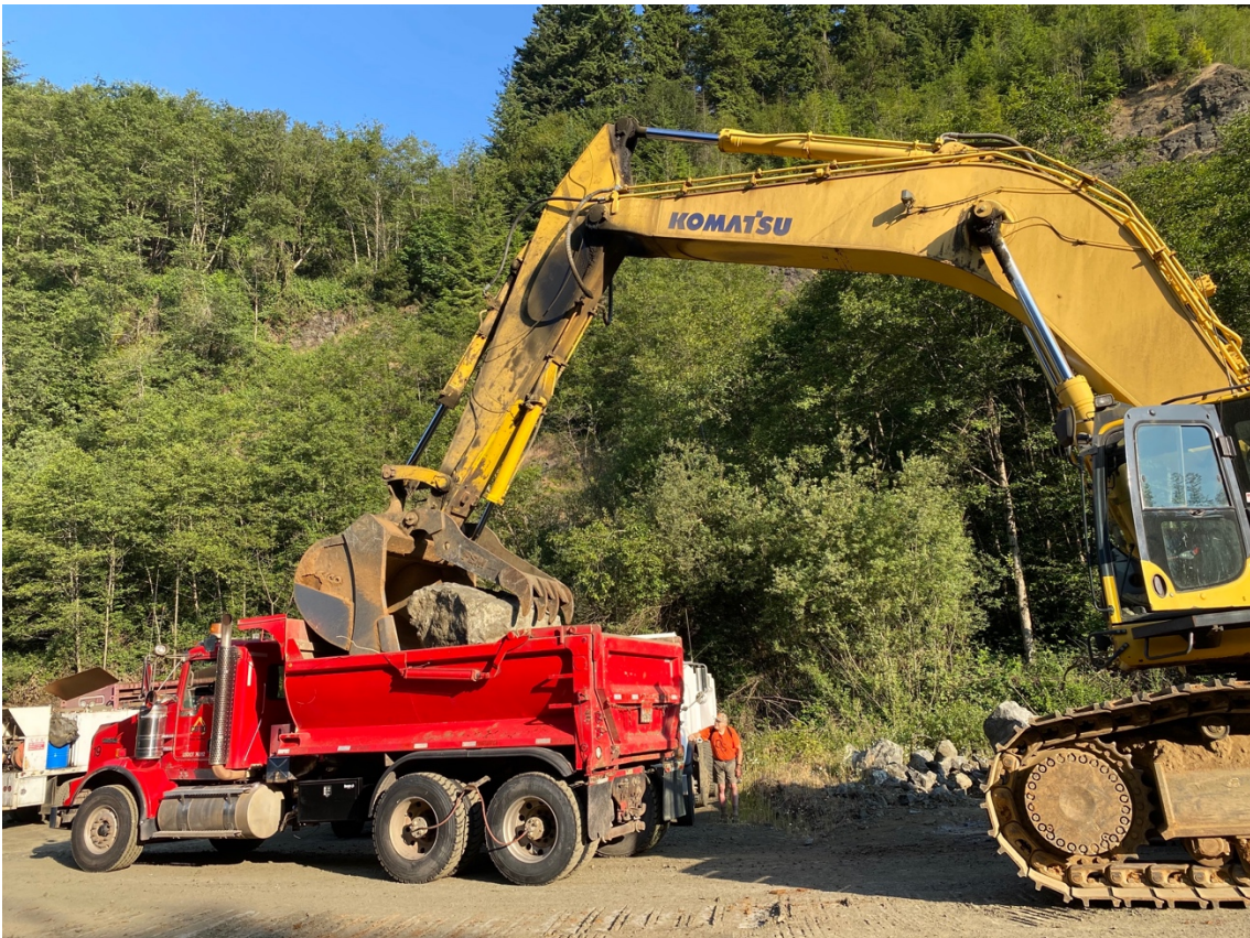
Main Rock's Komatsu PC800 depositing Memorial rock into bed of Coos Bay Timber Operators Kenworth dump truck, June 21, 2023. David Gould watches from background.
