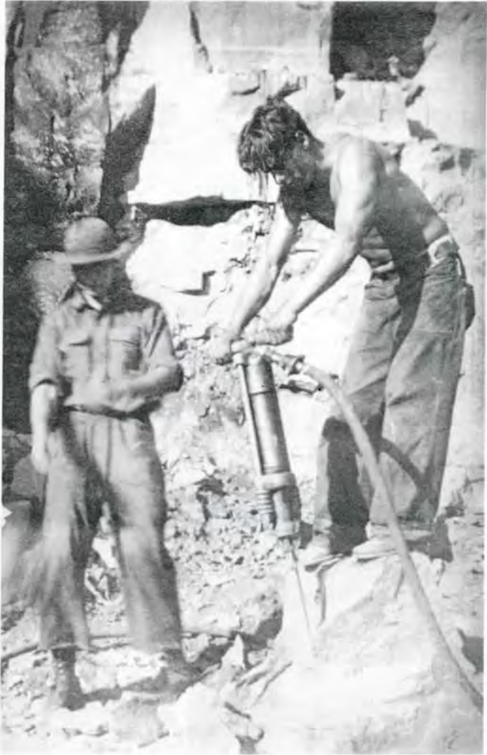
Sandstone rock drilling and blasting was a major activity during the construction of the Scholfield -Umpcoos Ridge Roads. Hardhats were unknown, but some wore "pith helmets" such as this man has. Surprisingly, injuries were uncommon. —Photo courtesy C.F.P.A. files
