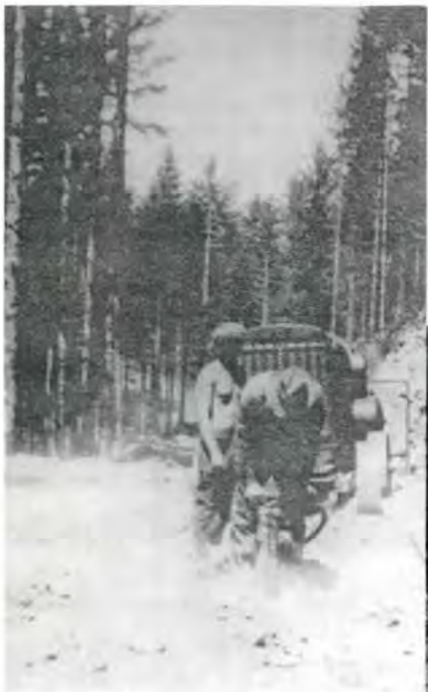
The 22 miles from Camp Walker to the junction with the Loon Lake Road was considered the toughest, rockiest construction of any CCC project in Oregon.
