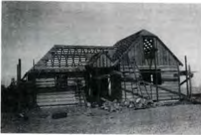
CFPA new office (1936) under CCC construction. This is the core part of the present CFPA Headquarters Office in Coos Bay. It was built by a side camp crew working out of Camp Walker, and, later, Camp Reedsport.
