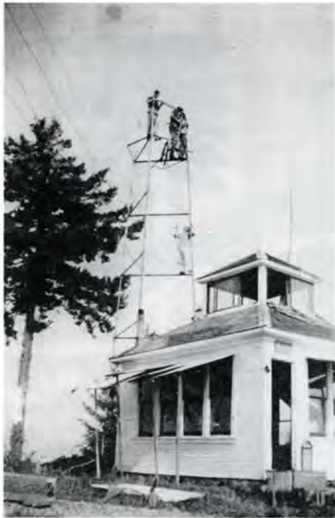
Between August of 1939 and July of 1940, CCCs built a 20-foot lookout tower, a 3-room cabin, and a woodshed on Dean's Mountain. It's interesting to wonder what today's safety standards would call for in the work shown here. —Photo courtesy of Inez Miller, Bandon.
