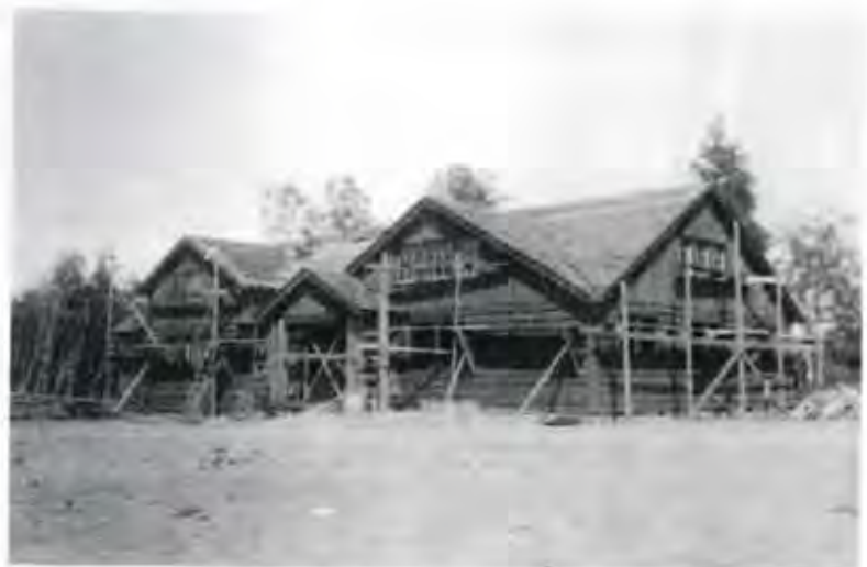
CFPA new warehouse (1936) under CCC construction. The CCC men first built what is now the warehouse and lived in it while they built the other buildings.
