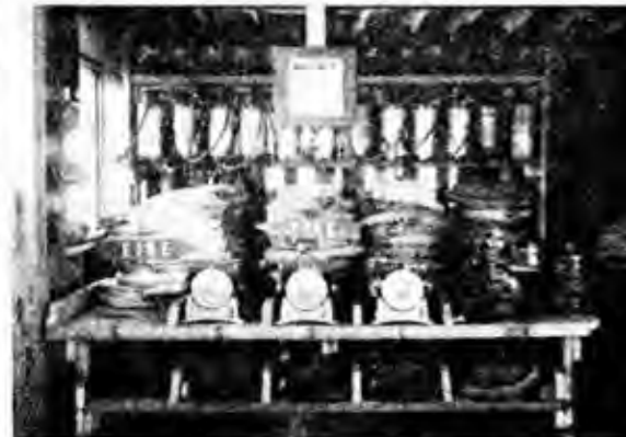
HOSE AND PORTABLE PUMPS ALWAYS READY FOR ACTION
