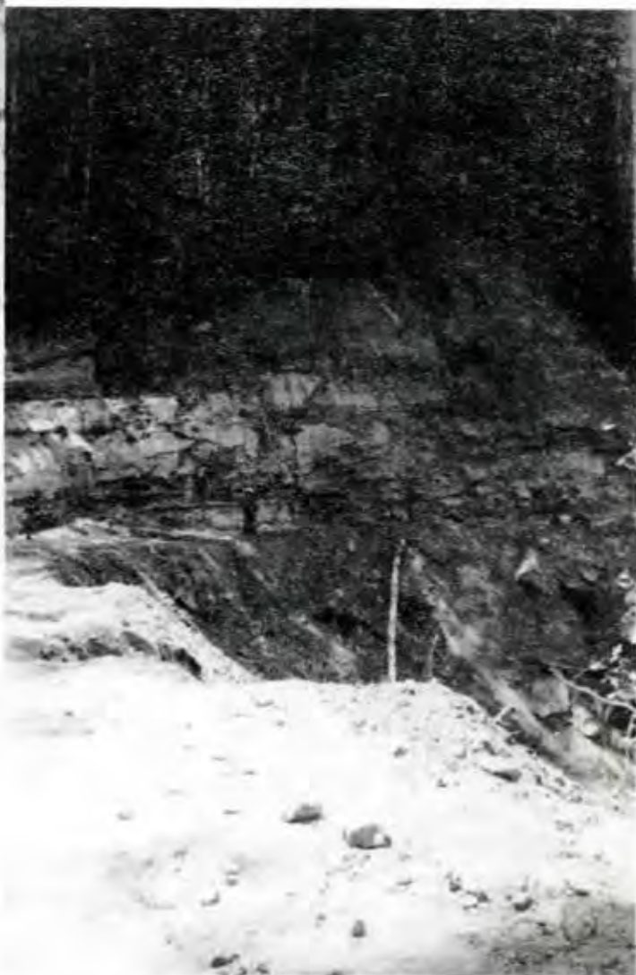
Typical tough road construction by CCC crew on Elliott Forest. — Photos from Coos Forest Protection Association files.
