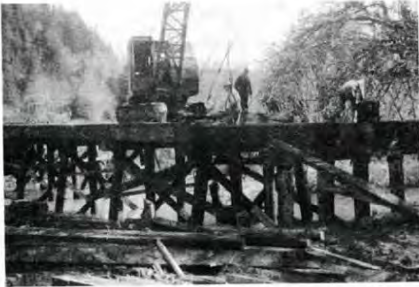
Lake Creek Bridge under construction in August, 1961, Contractor Sig Anderson, for the Al Peirce Company. Photo courtesy of George Shore
