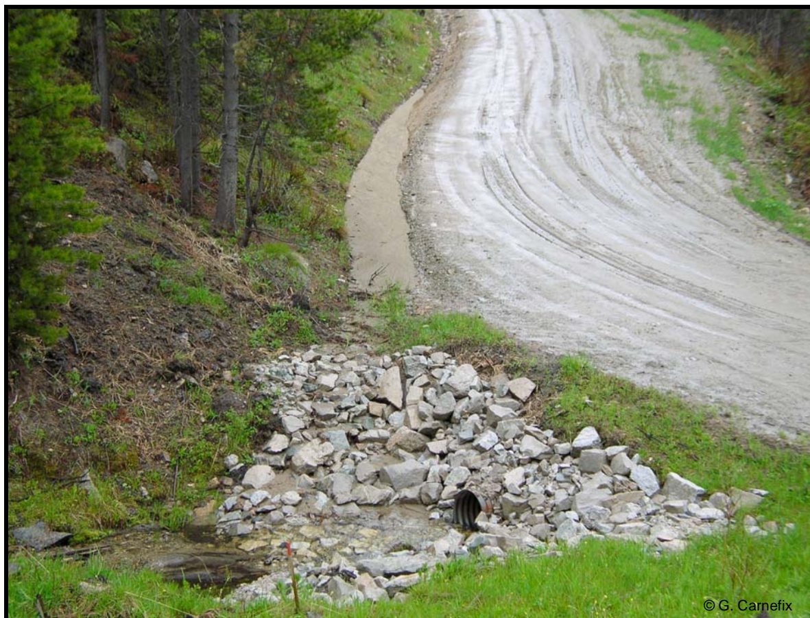
Photograph 1. An example of an ineffective Best Management Practice (BMP) that failed to significantly reduce major impacts of land use on aquatic systems on the Bitterroot National Forest, MT. High levels of fine sediment from road impacts continue to be funneled directly to this stream via road drainage features, despite the recent addition of rock to the stream crossing in 2005. The stream is in the East Fork of the Bitterroot River watershed, which is designated as having impaired water quality due to sedimentation. This watershed provides habitat for bull trout, listed as threatened under the Endangered Species Act, and imperiled western cutthroat trout. Increases in fine sediment significantly reduce the survival of both these native trout, as discussed in the text. Photograph: G. Carnefix.
