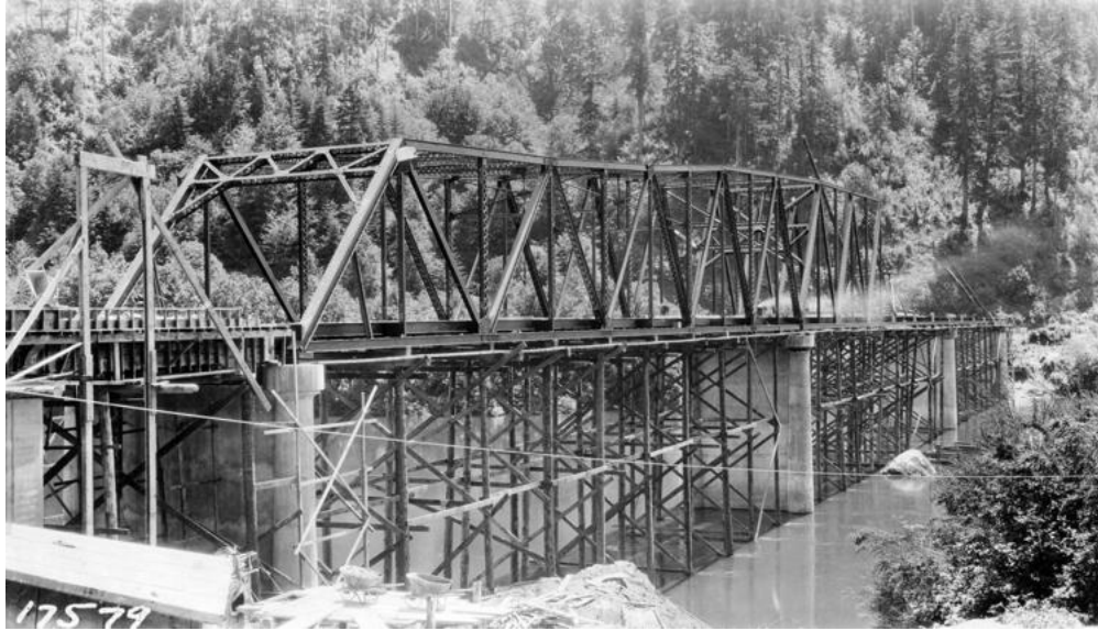
The Scottsburg Bridge sits across the Umpqua River partially completed in 1929. Pre-construction on a new bridge to replace the aging structure will begin in February.
